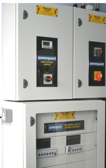
WIND TURBINE & CHP CONTROL
