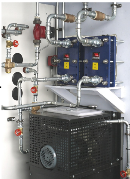
HEAT DUMP & OUTPUT HEAT EXCHANGERS
