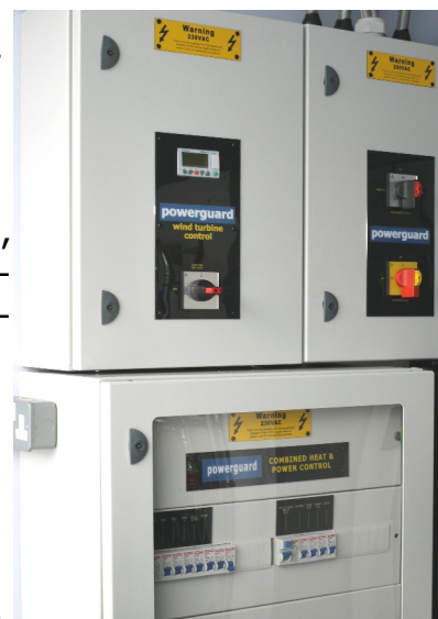
WIND TURBINE & CHP CONTROL
