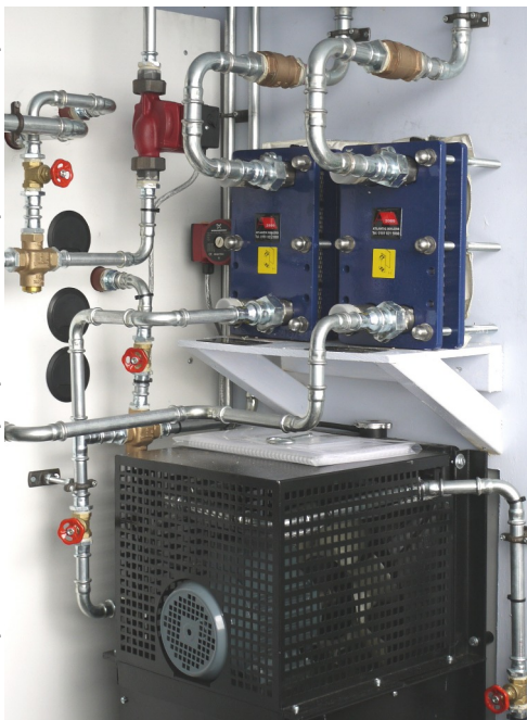
HEAT DUMP & OUTPUT HEAT EXCHANGERS
