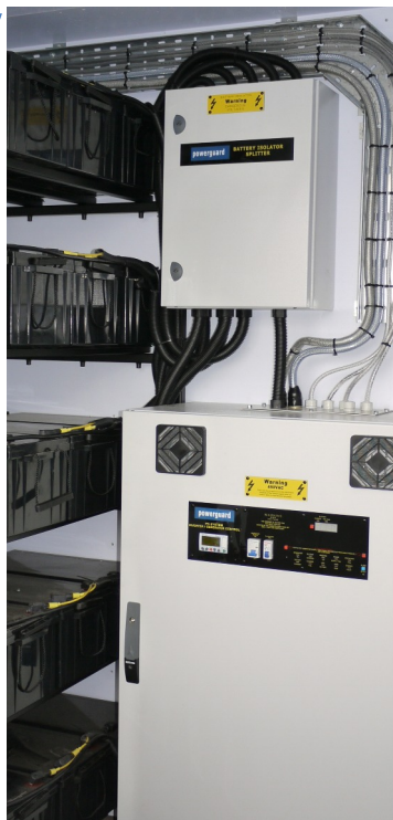
PS SYSTEM & BATTERIES
